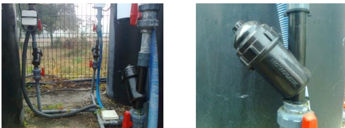
Figure 33 Filter distribution installation (left) and filter detail (right)
