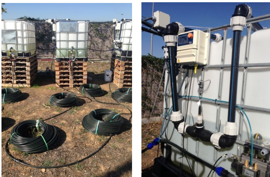
Figure 6 View of 400-m pipeline and storage tanks (left) and detail of chlorination system installed in tanks 501 and 503 (right)
