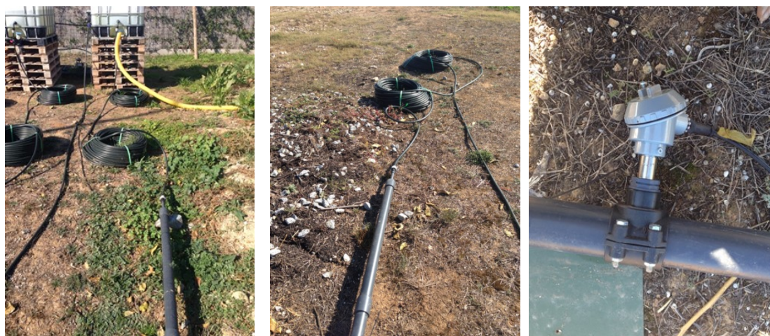
Figure 13 Installation of PVC pipe to the pilot pipe 504 and mounted ALVIM sensor (right)
